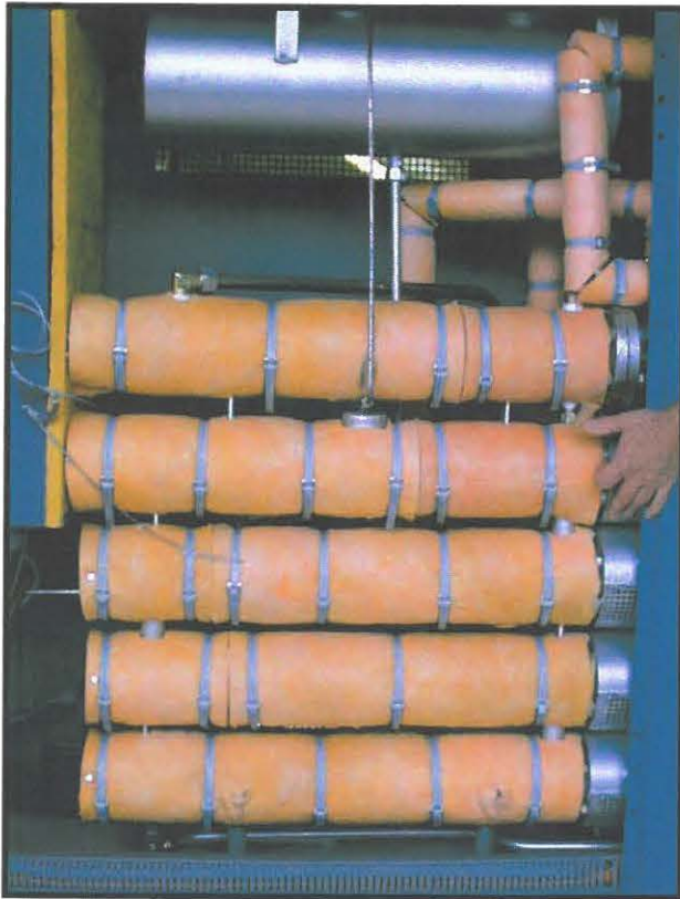
Expansion tank, Heat exchanger, and four heating elements
