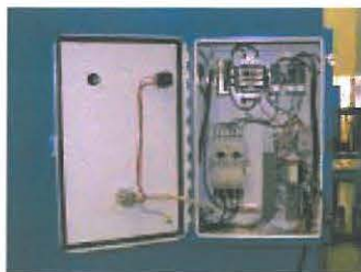
Casting Cooler Control Panel
